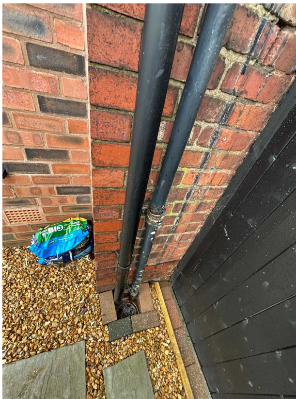
Base of RWP to porch roof
