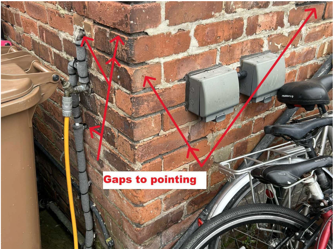
Gaps to point, rear low level
