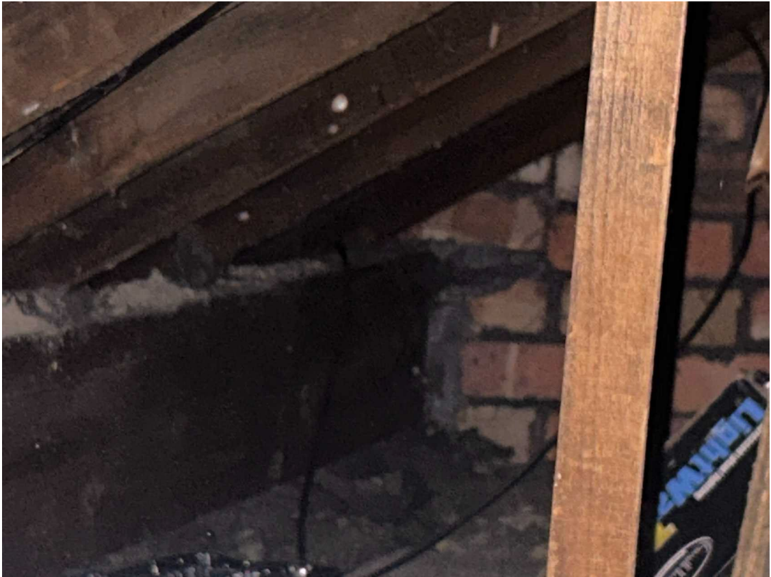
View to purlin support below hole in the roof
