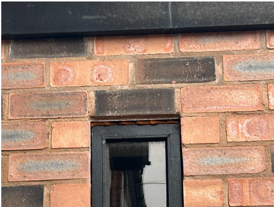
Typical window to porch, missing sealant
