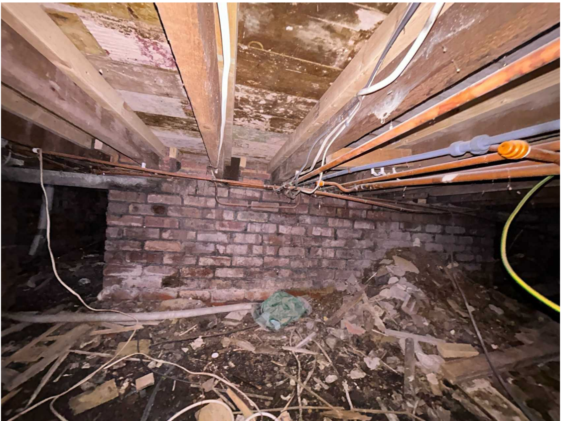
View to floor void- note debris
