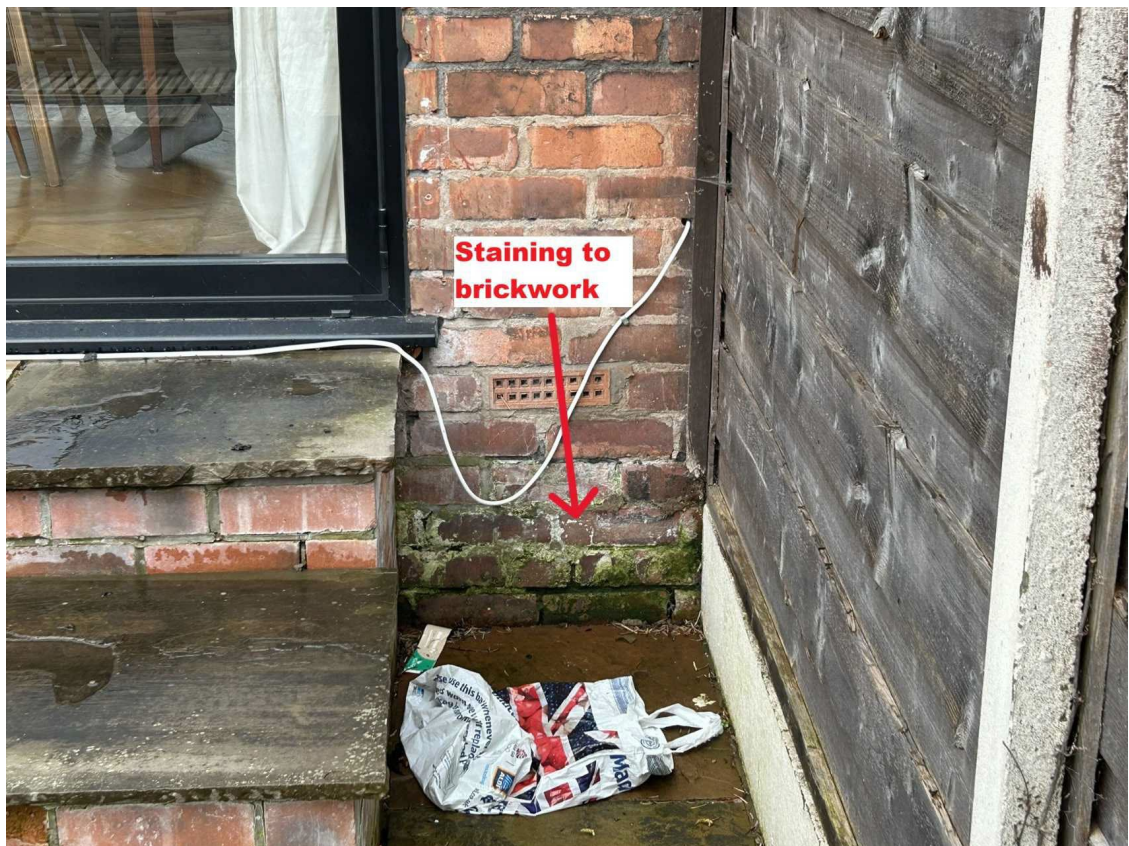
View to staining due to water ponding to paving
