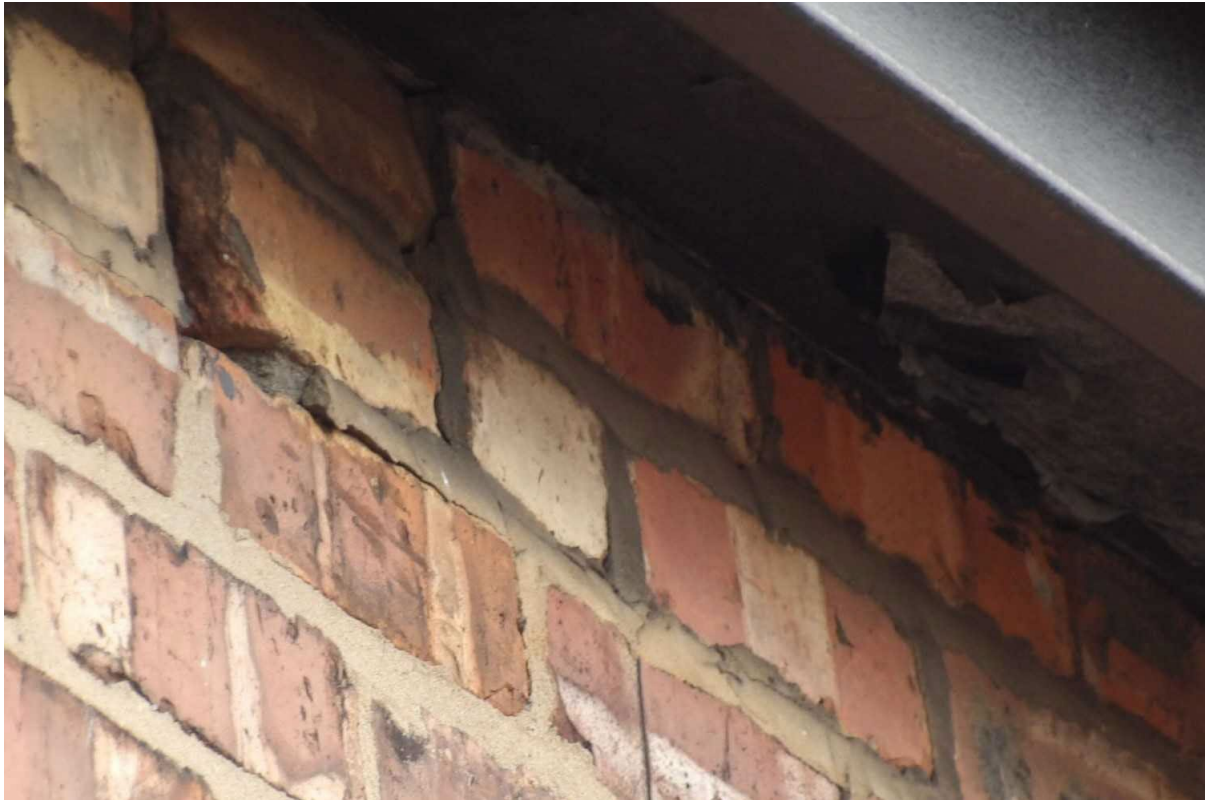
View to damage brickwork to gable
