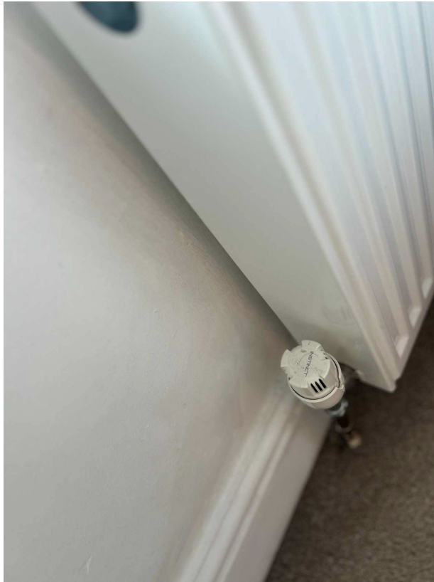
Valve to radiator
