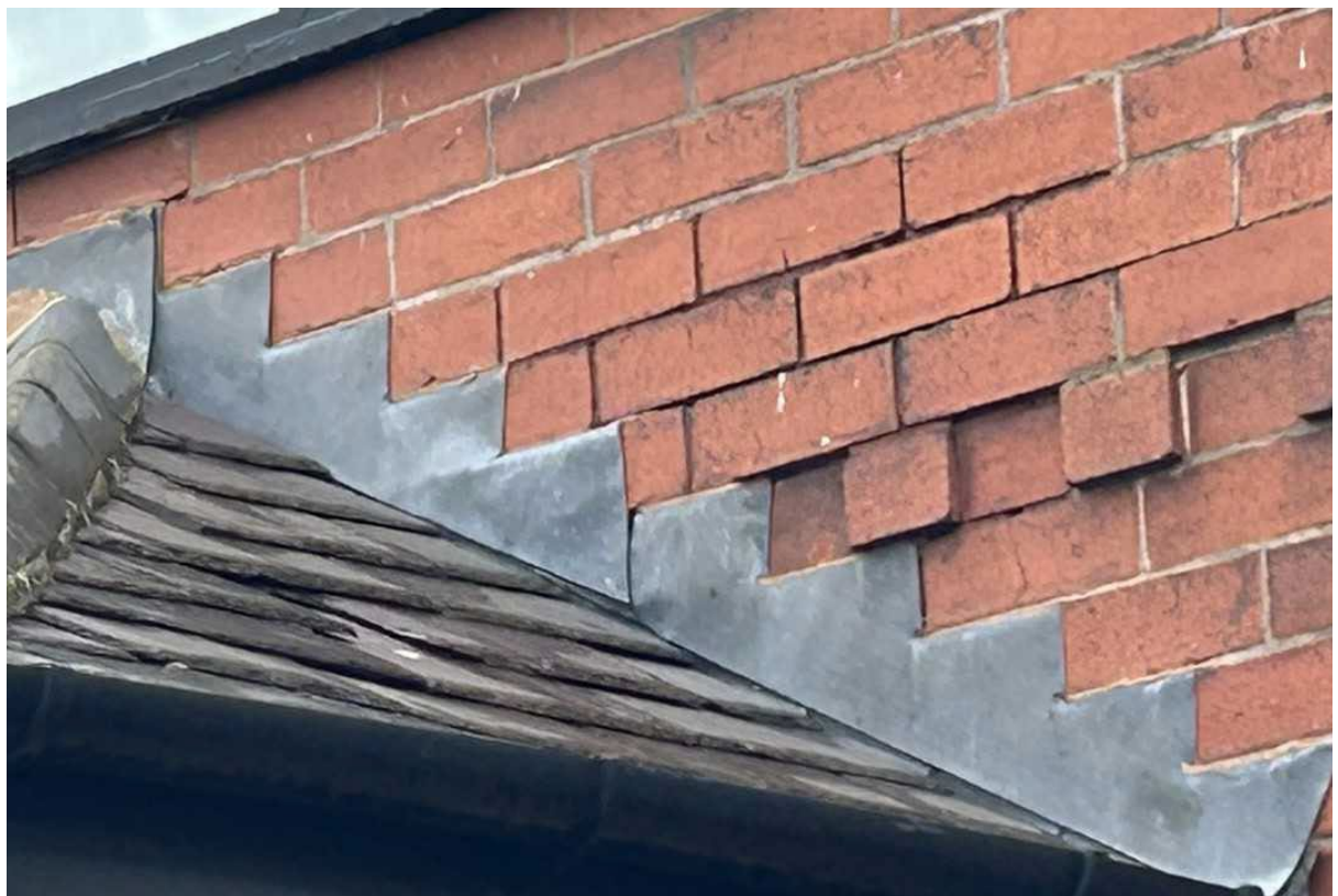
View to gaps to pointing above porch
