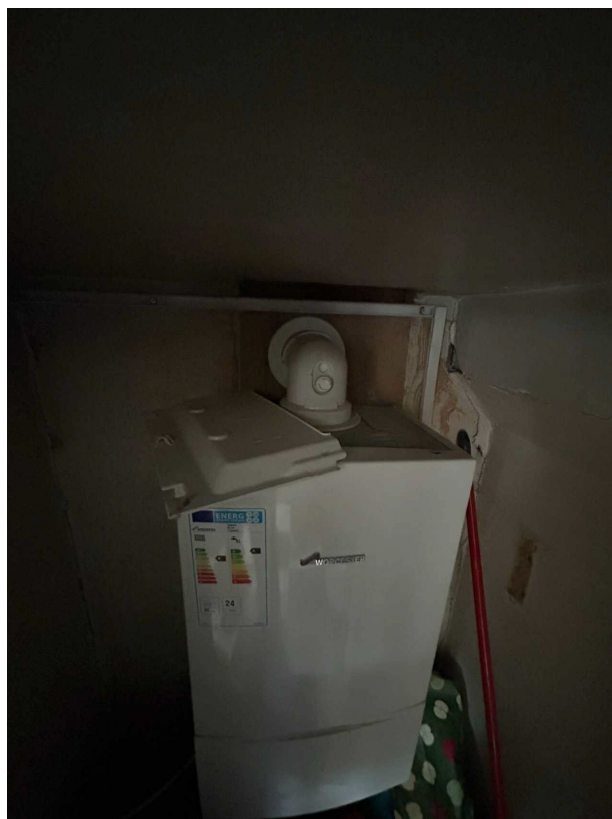
Flue to boiler
