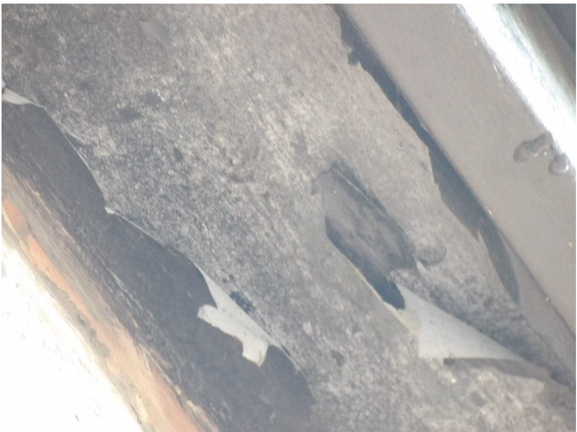
Peeling paintwork to soffit on the right hand side
