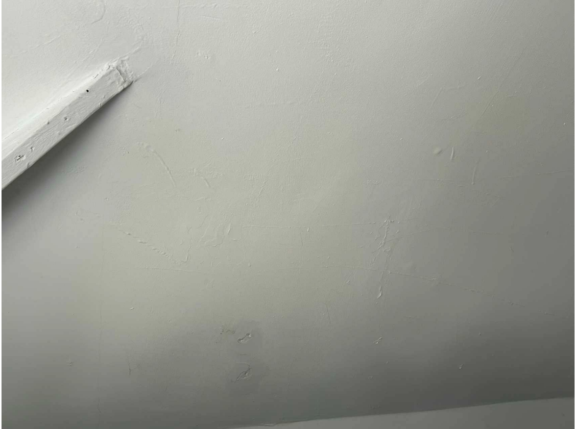
Bedroom 3- rough finish to ceiling
