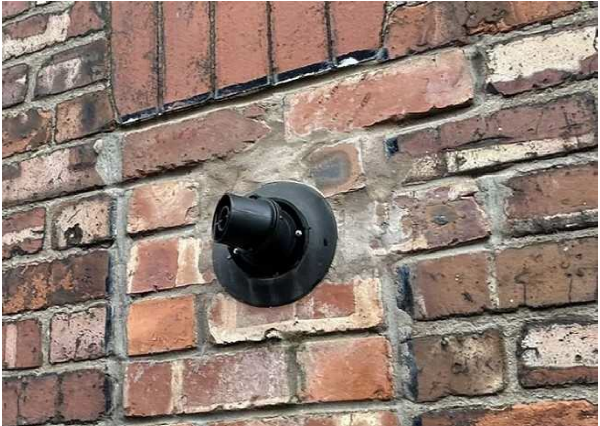
View to boiler flue
