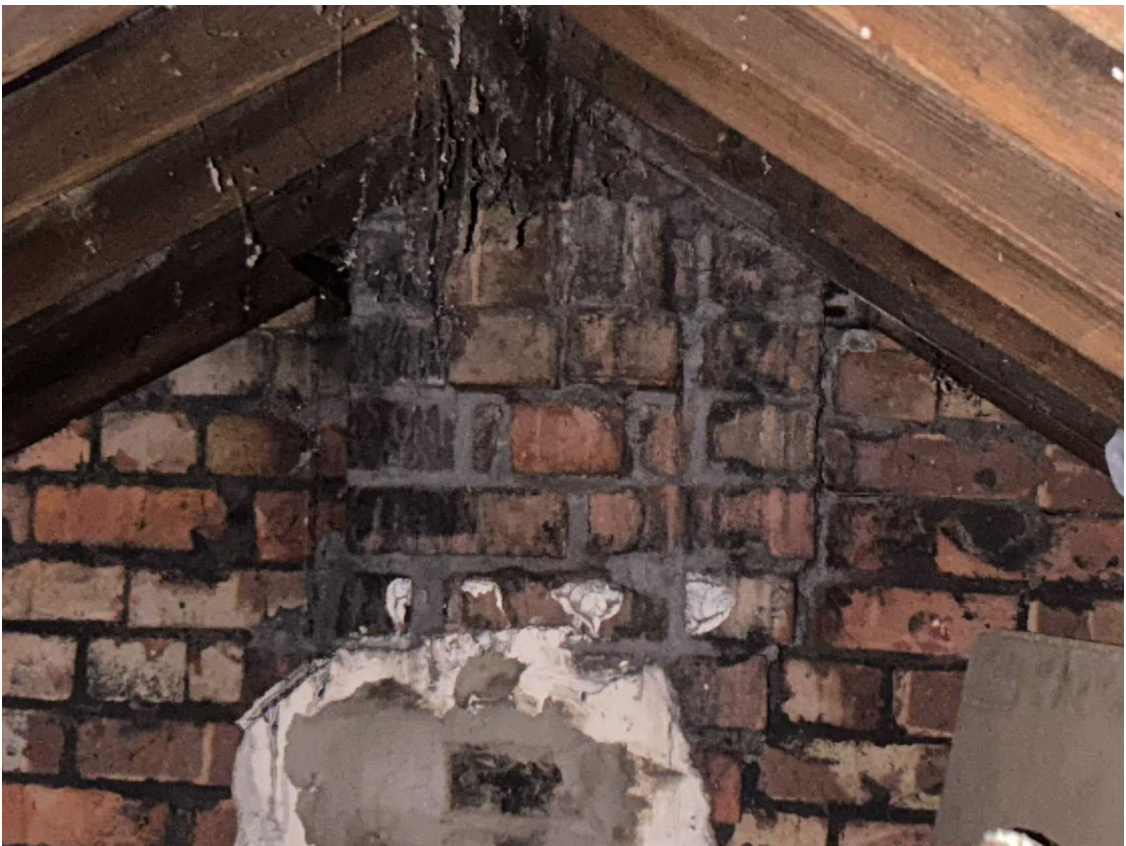
View to party wall - staining to chimney breast
