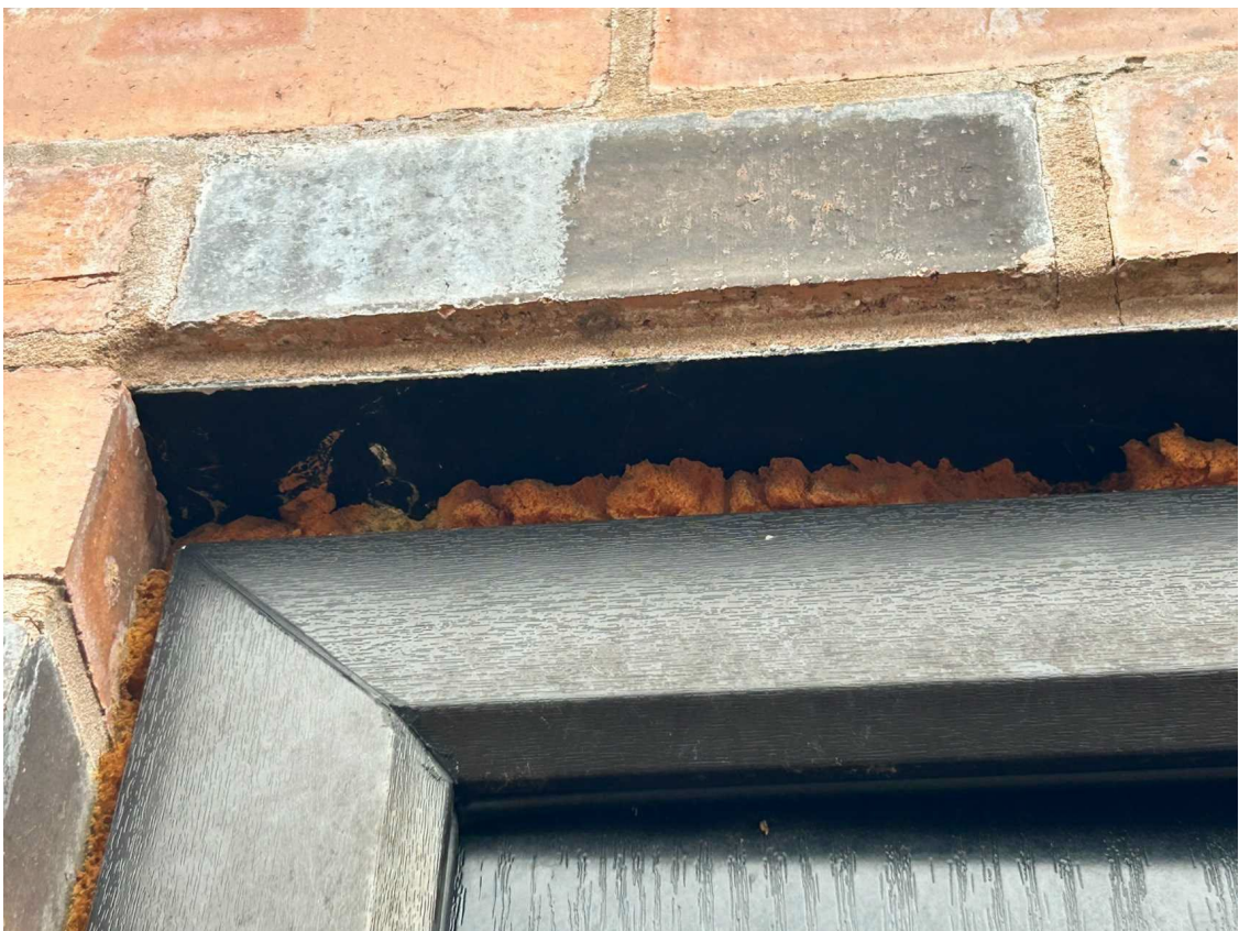
Missing sealant to front door
