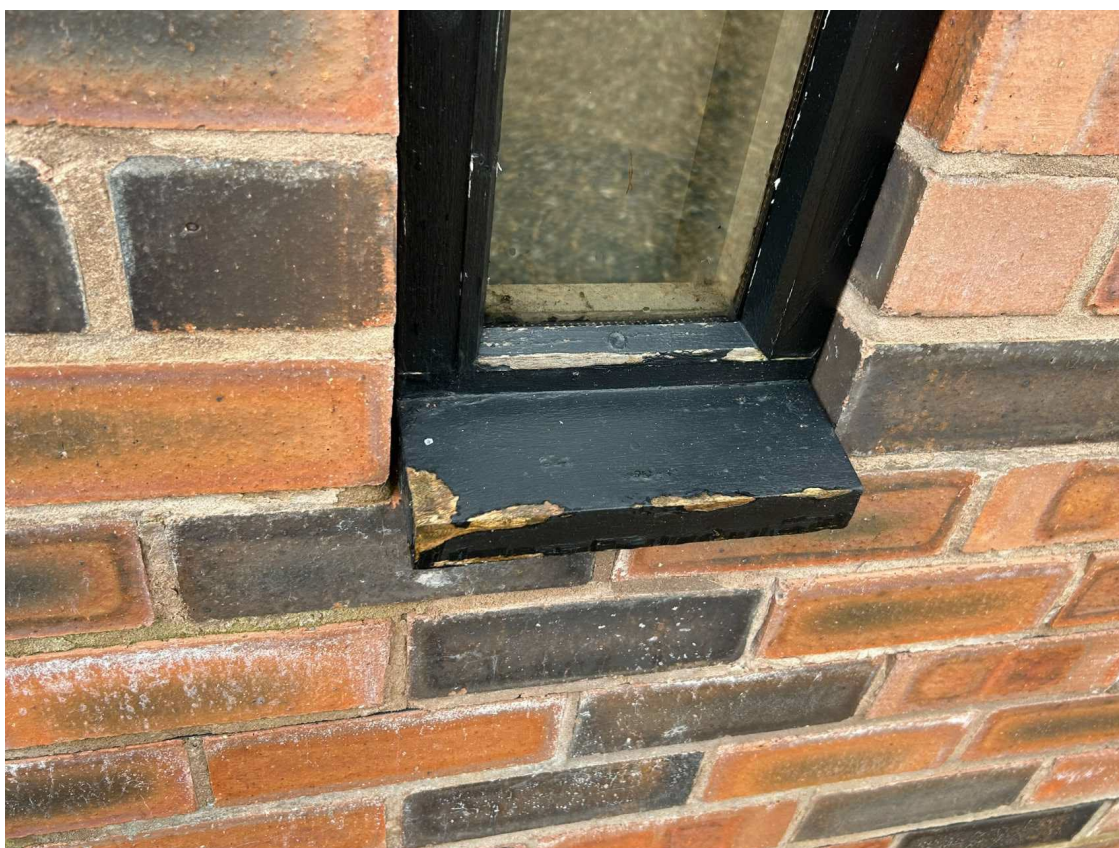
Porch window, damage to cill.
