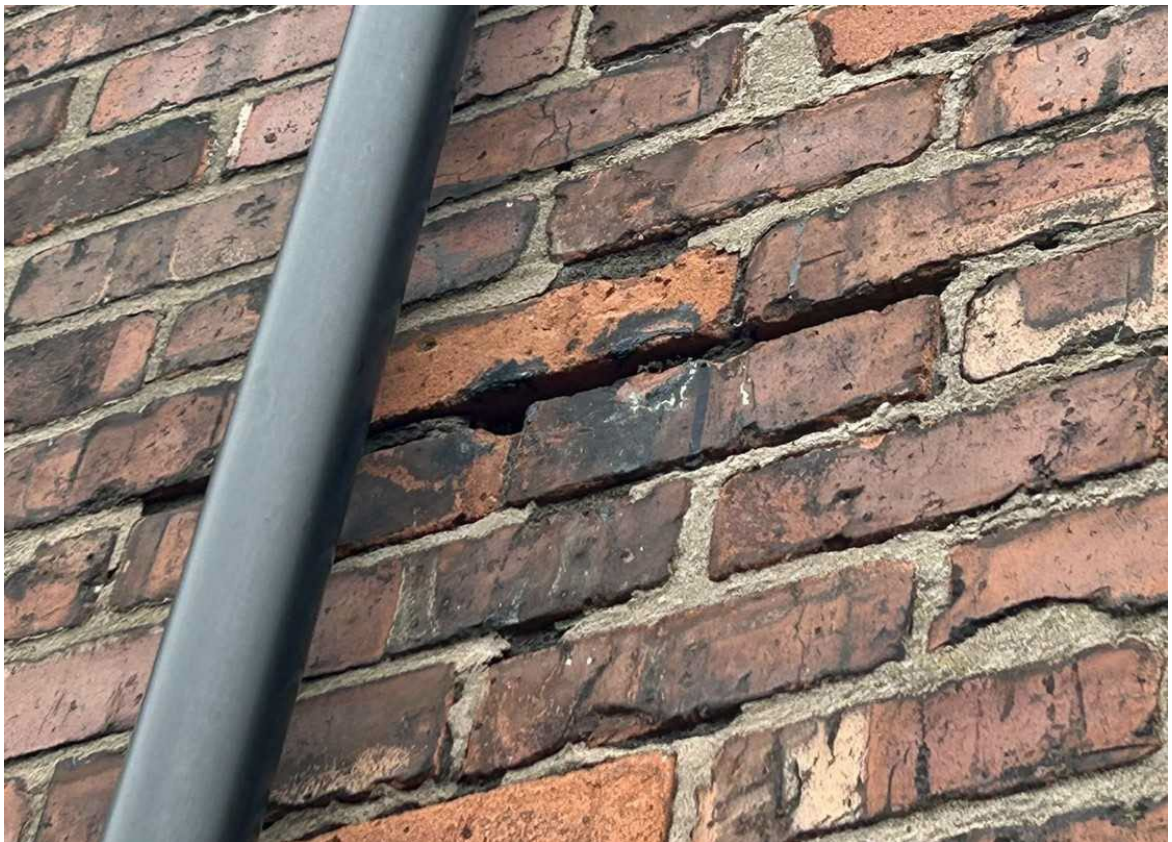
View to typical gaps to brickwork to gable
