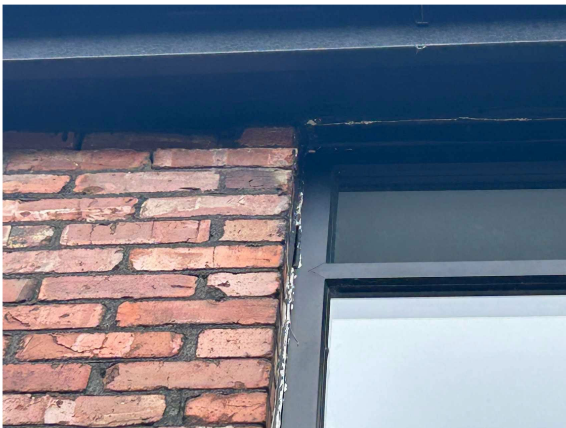
Gaps to sealant- rear windows
